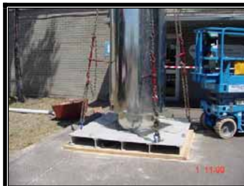
NAC-LWT Cask Loading Area
