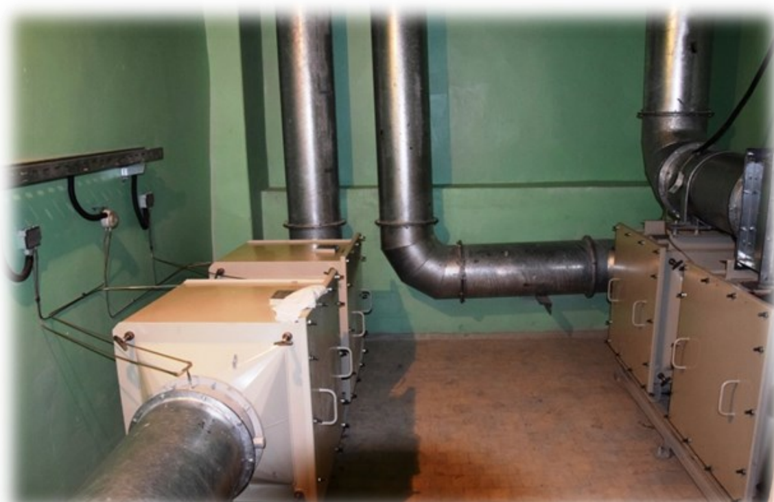
Fig. 2. Exhaust ventilation and filtration system
