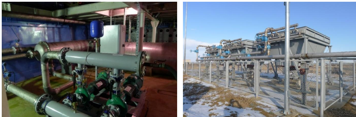
Figure 2. Cooling system for the primary coolant of the IVG.1M reactor a) Heat exchanger and pumps premise; b) Chillers
