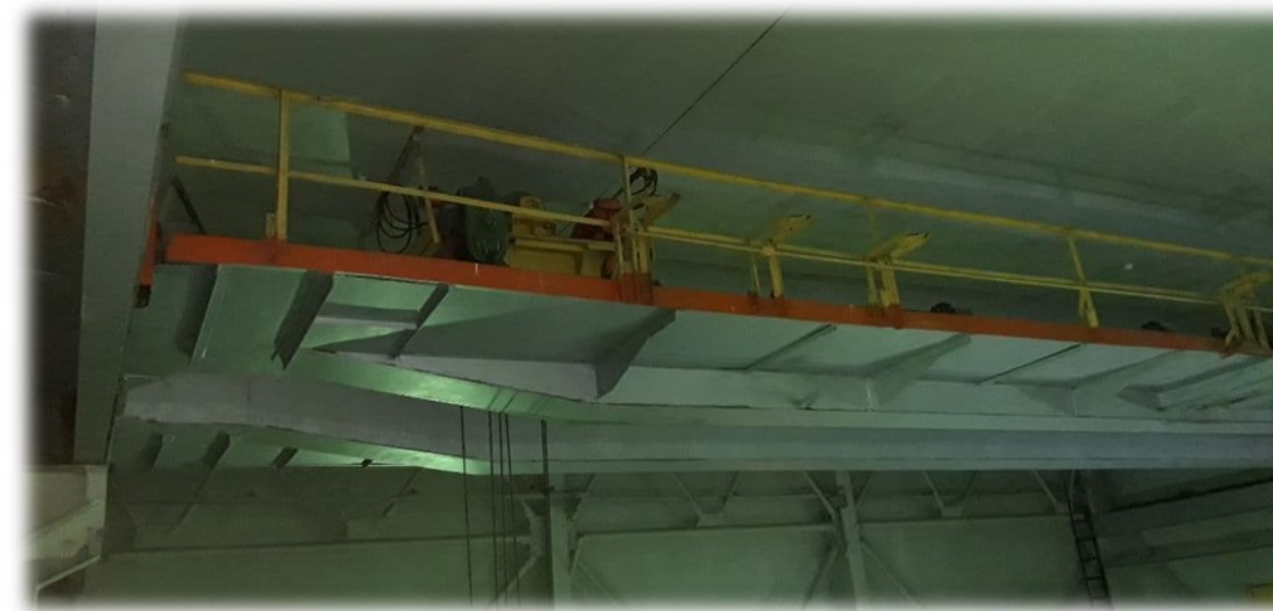
Fig. 4. 10-ton overhead crane
