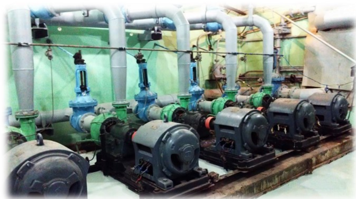
Fig. 3. primary cooling system pumps
